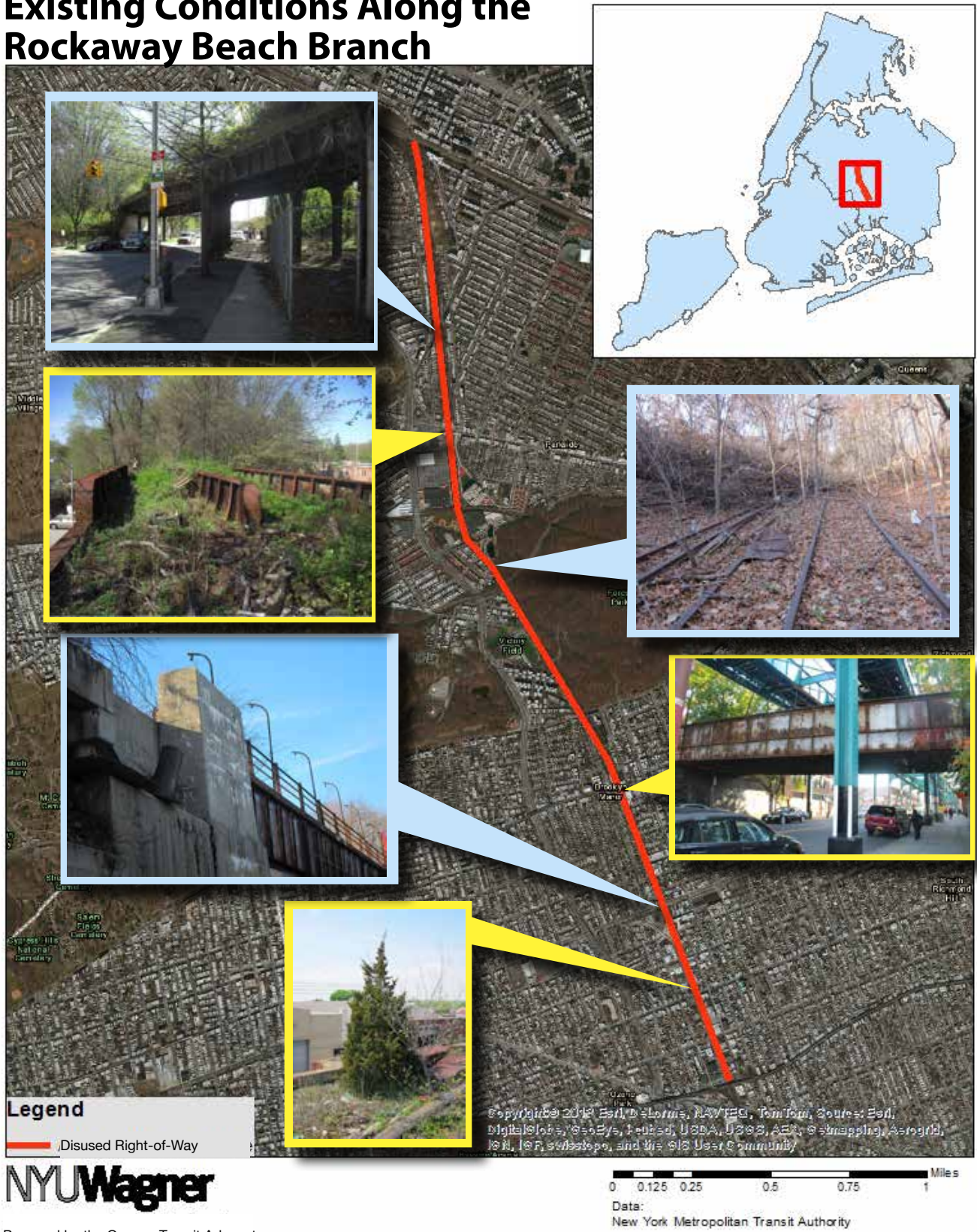
Figure 3 (above) shows existing conditions at various points along the disused portion of the Rockaway Beach Branch. While the right-of-way remains intact, the infrastructure itself remains in various states of disrepair.
