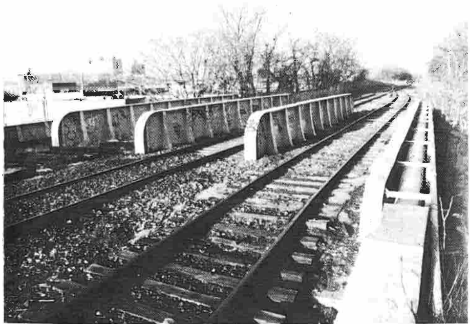
Space for four tracks on the bridge over Remsen Ave. in East Flatbush. A station for the Brooklyn Terminal Market could be located here.
